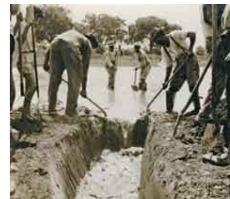
Early efforts of 'vector control' by workers somewhere in the US in the 1920s. Digging a drainage ditch removed standing water, the breeding ground for mosquitoes transmitting malaria and dengue fever.
